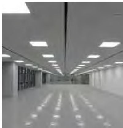
Highly efficient LED lighting
